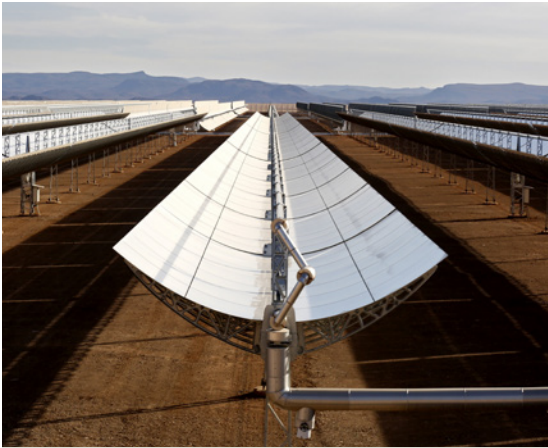
Solar panels of the mega solar plant of Ouarzazate, in southern Morocco, built by a Spanish consortium.
