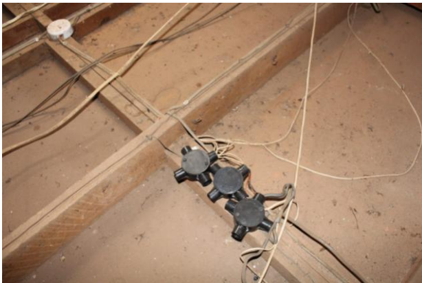
Exposed electrical installations
