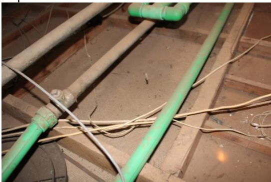
Metallic water pipes
