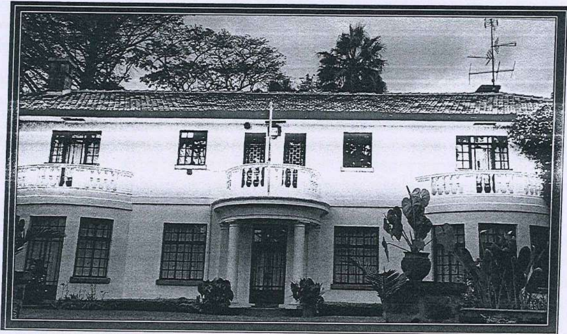
Picture 2: Back view of the earmarked house whose ceiling will be removed then reroofed and renovated.
