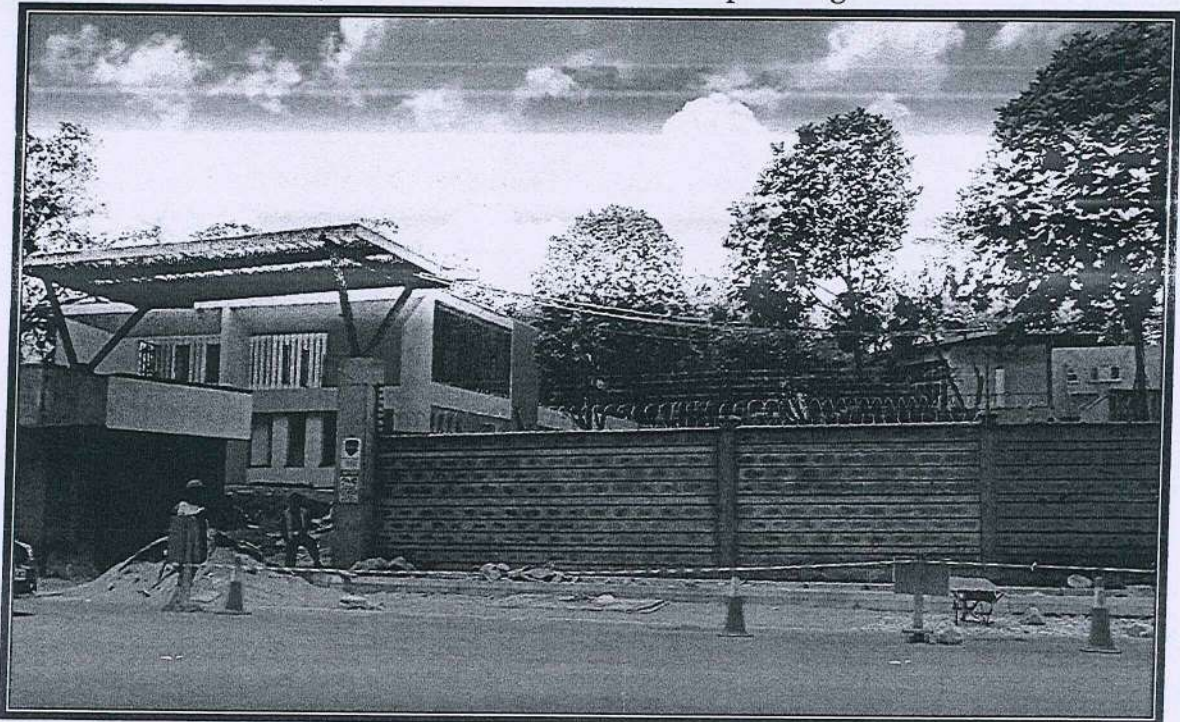
Picture 7: Some of the few up-market residential maisonettes under construction in this quiet neighbourhood, along Gatethuru road.
