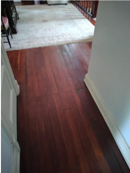
Timber deck flooring-Sanding needed
