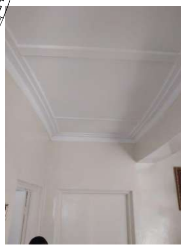
Existing ceiling in the corridor. All new ceiling works to mimic the same
