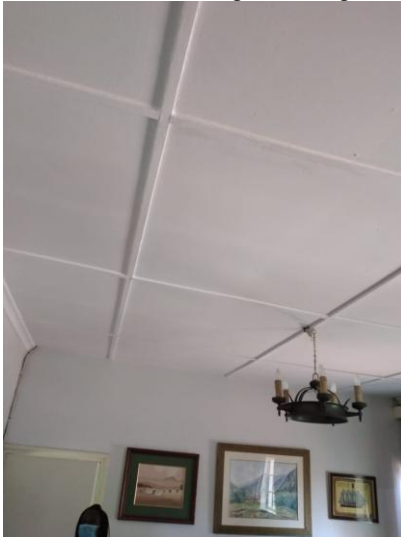
Asbestos ceiling in the bedrooms
