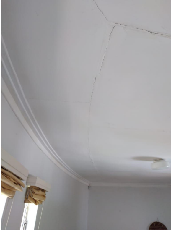
Cracked slab ceiling in the kitchen
