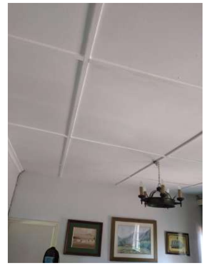
Existing ceiling in the bedrooms. All new ceiling works to mimic the same
