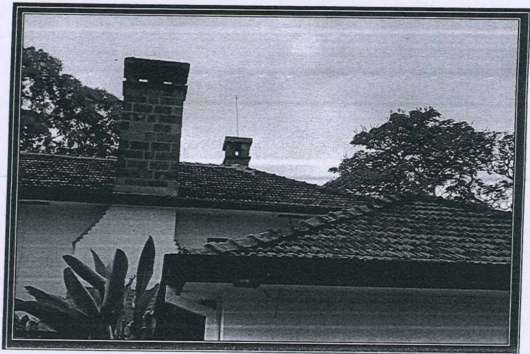
Picture 6: The current condition of the roof, to be renovated, underneath of which the asbestos ceilings exist.
